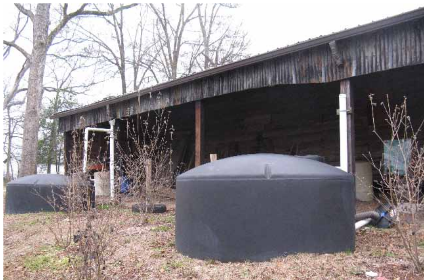
Two large above-ground cisterns collect rainwater falling on the doctor's office roof at Pioneer Park.
